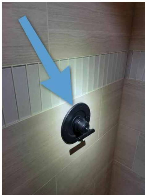
Escutcheon plate(s) missing seal.
