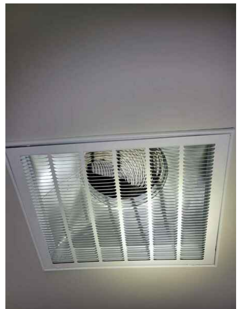
Return air register did not have a filter.
