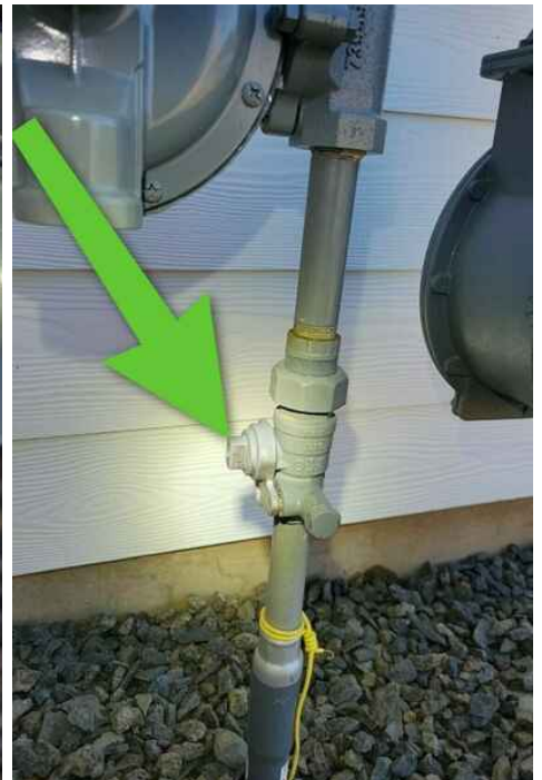
Main utility shutoff valve.
