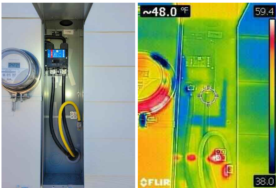
Thermal image scan for overheating breakers: Normal
