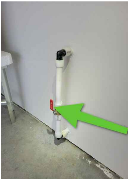
Main water supply pipe in garage with shut-off valve.
