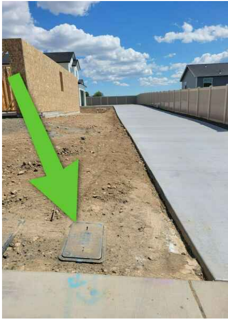
Water meter location.
