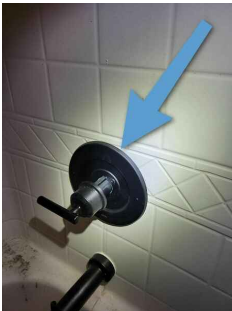
Escutcheon plate(s) missing seal.
