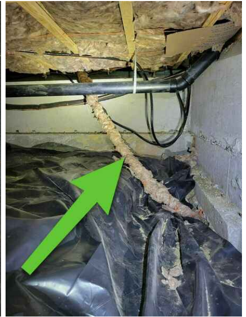
Main water supply pipe. Southwest crawlspace.
