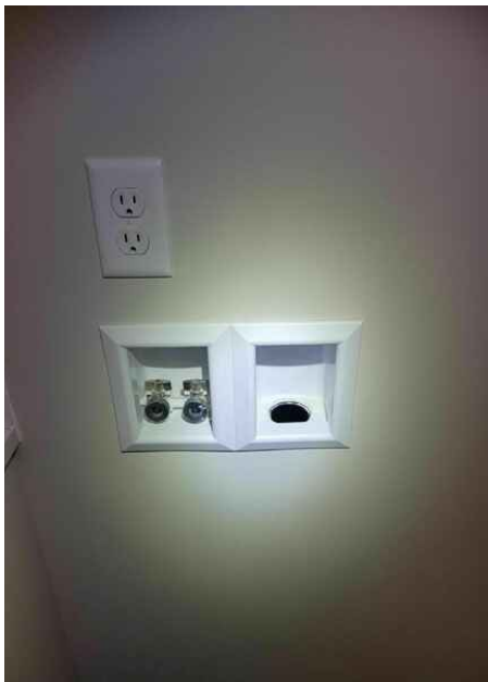
Water supply pipes/valves and drain pipe.
