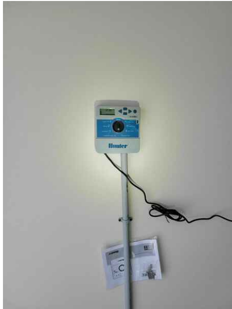
Control hub. Garage.
