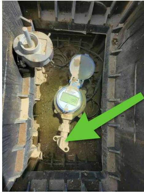
Water meter with main shut-off valve.
